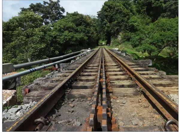
Rack & pinion system tracks
