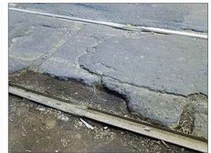
▲ Broken tram tracks various places along M G Road
