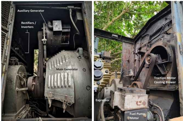
Generator Compartment of a YDM-4
