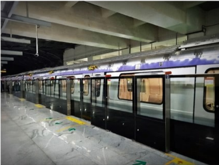
Platform Screen Doors (PSDs)
